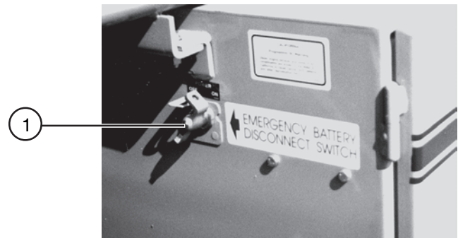
Figure 2-2. Emergency Battery Disconnect Switch
